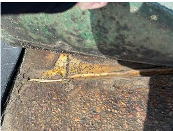
Figure 1 - Beneath Rubber Pavers, Mold, mildew, ants
