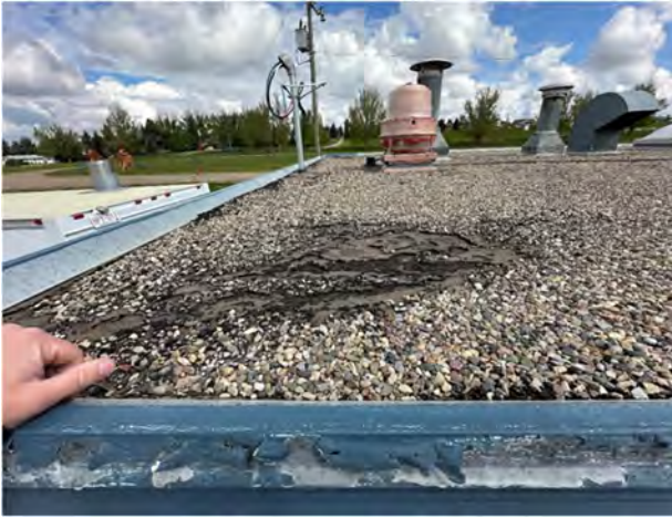
Figure 13 - Deteriorated Roofing Material
