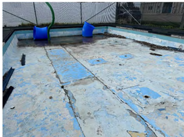
Figure 2 - Cracking/Spalling of the small pool basin
