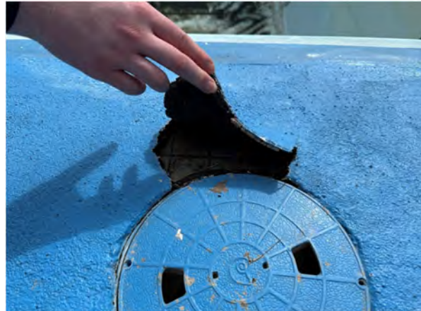
Figure 10- Peeling Rubber Surface
