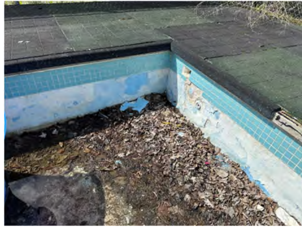
Figure 4- Debris Collecting in basin, leading to staining
