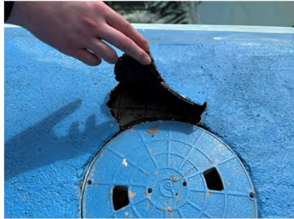
Figure 6- Peeling Rubber Surface
