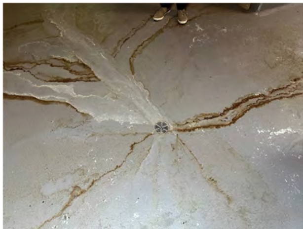
Figure 12- Water Stained Floors from Roof Leaks
