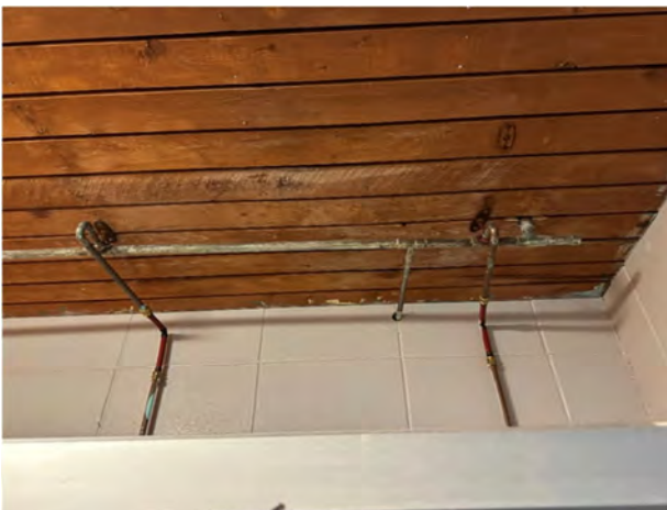
Figure 11 – Water Damaged Ceiling Slats
