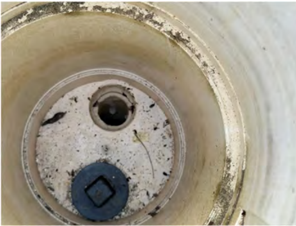
Figure 7 –Cracked Skimmer Drain
